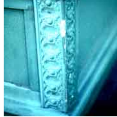
Substitute materials need to be located with care to avoid damage. The fiberglass column base has chipped, whereas the historic cast iron would have remained sound. Photo: NPS files.
