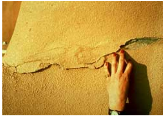
A waterproof coating is an inappropriate substitute material to apply to adobe as it seals in moisture and may result in spalling. Photo: NPS files.
