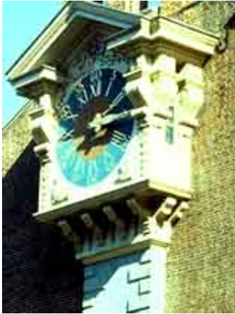
In the reconstruction of the clock tower at Independence Hall, the substitute materials used were cast stone and wood with fiberglass and polyester bronze ornamentation. Photo: NPS files.
